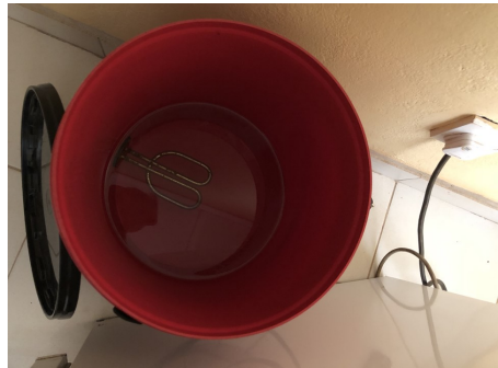
A plastic bin with a heating element installed - don't overheat!
