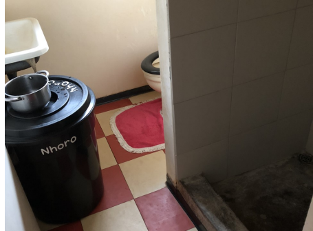
A washroom with toilet, sink and shower but no running water
