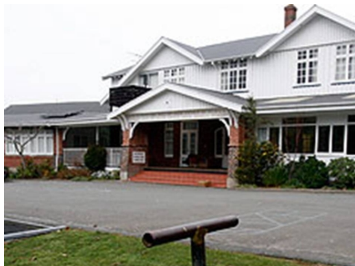
A 2011 Earthquake left a big crack through the middle of Cholmondeley Children's Home
